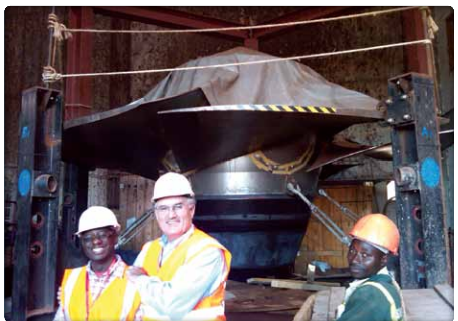
Five 51 MW Kaplan turbine-generator units were installed in the powerhouse of the 250 MW Bujagali project in Uganda, the largest private sector investment ever undertaken in the region.
